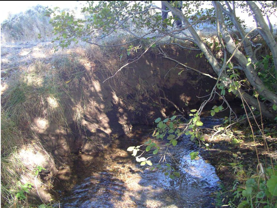
Figure 5: Approximately 3 feet high cutbank eroding the north bank, in an aspen grove. Photograph taken at approximately station 50+00, view is facing upstream.
